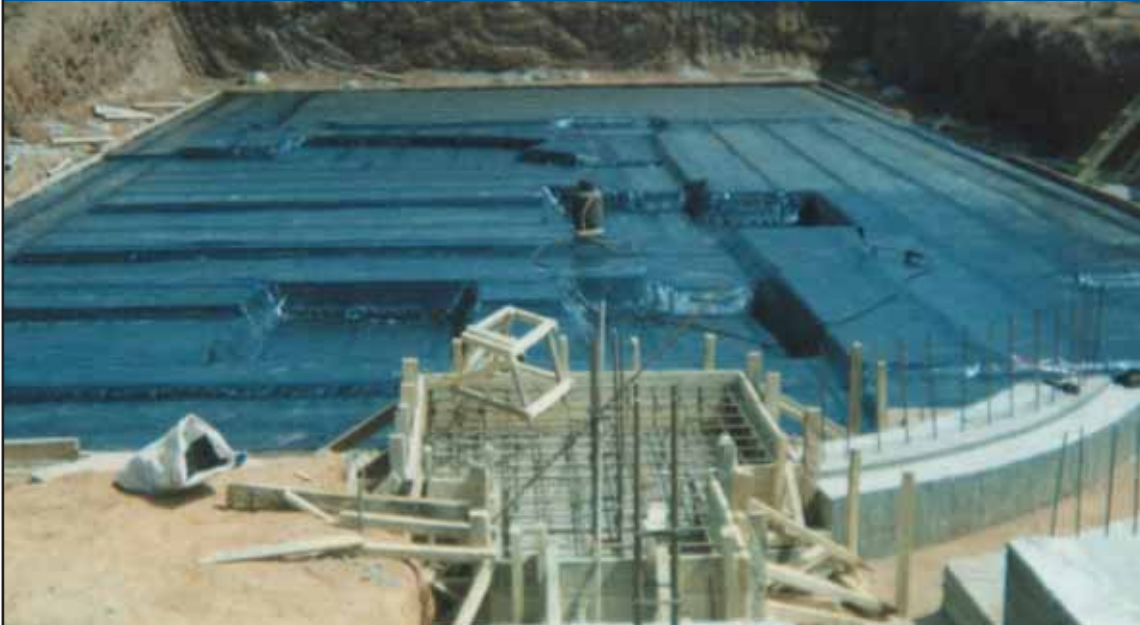
Substructure protected with Denso 3000 SA waterproof membrane. Tanking supplied and applied by MasterProofer Ltd, Lagos.
