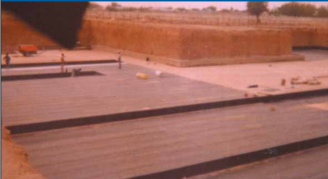
Substructure protected with Denso 3000 SA waterproof membrane. Tanking supplied and applied by MasterProofer Ltd, Lagos.
